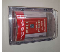
Lobby Pull Station
